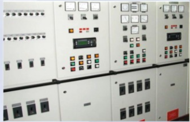
ELECTRICAL PANEL INDUSTRY
