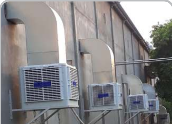
Factory & Heavy Industries Cooling
