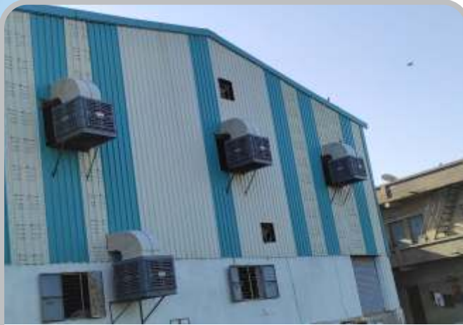
Engineering Industries cooling
